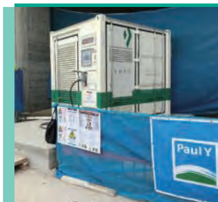
The Group has introduced "Enerstainer-Lithium-Ion Energy Storage System" at our construction sites which reduces noise and carbon emission during electricity supply. 集團於工地引進淨能櫃—鋰離子儲能系統，以減少提供電力時的噪音及碳排放。
